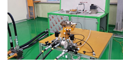
TBN Governor Actuator / ETS 계통 정비 시스템 (TBN Governor Actuator / ETS System Equipment)
